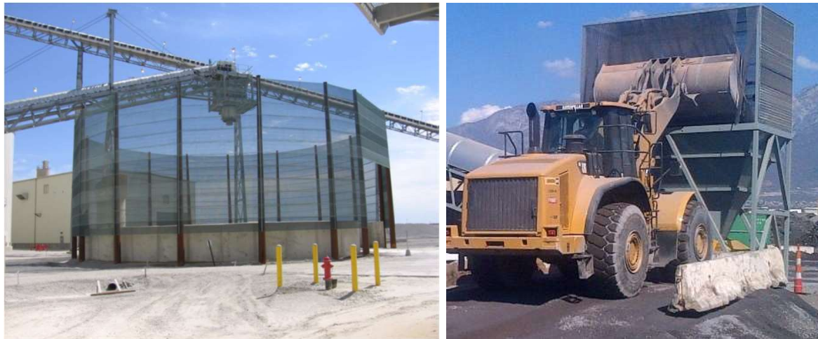
Figure 3.14. Typical wind fence installations. Left: porous windbreak material around stockpile drop. Right: material being used in loadout hopper.
