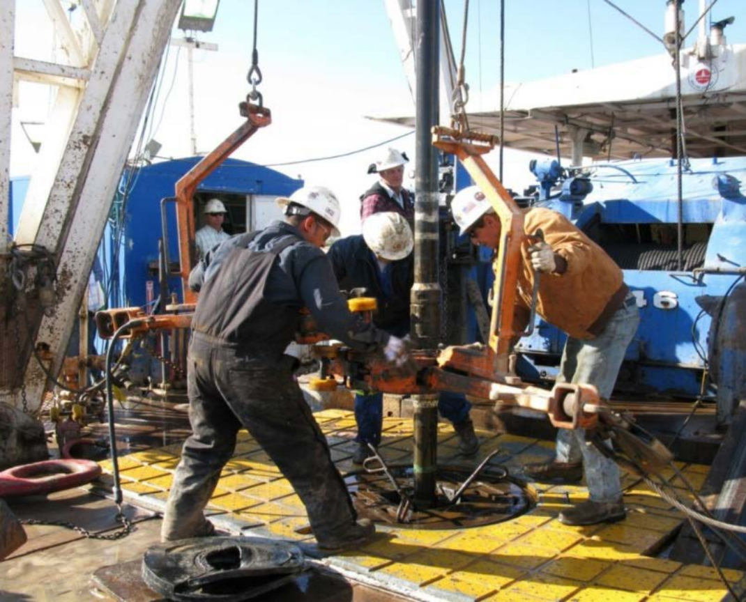
Drilling rig floor
